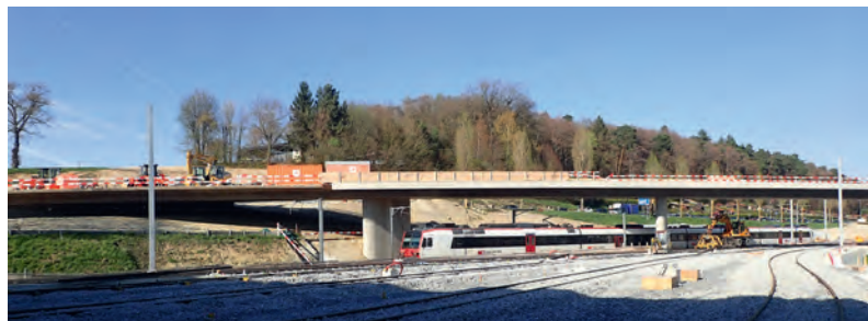
Fig. 7 Franchissement des voies et culée intégrale nord. Track crossing as well as integral northern abutment.
