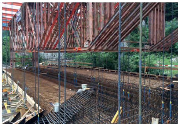
Fig. 8 Engagement des cintres par-dessus le tablier. Use of falsework over the bridge deck.
