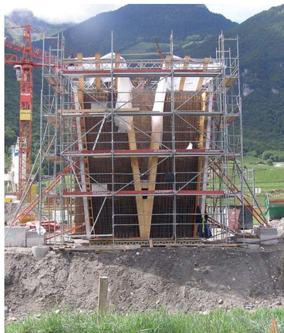
Fig. 5 Echafaudage, coffrage et armature d'une double pile. Scaffolding, formwork and reinforcement of a double pier.
