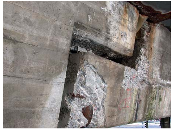
Fig. 3 Gravierende Schäden an Gerbergelenken. Serious damage to the Gerber hinges.
