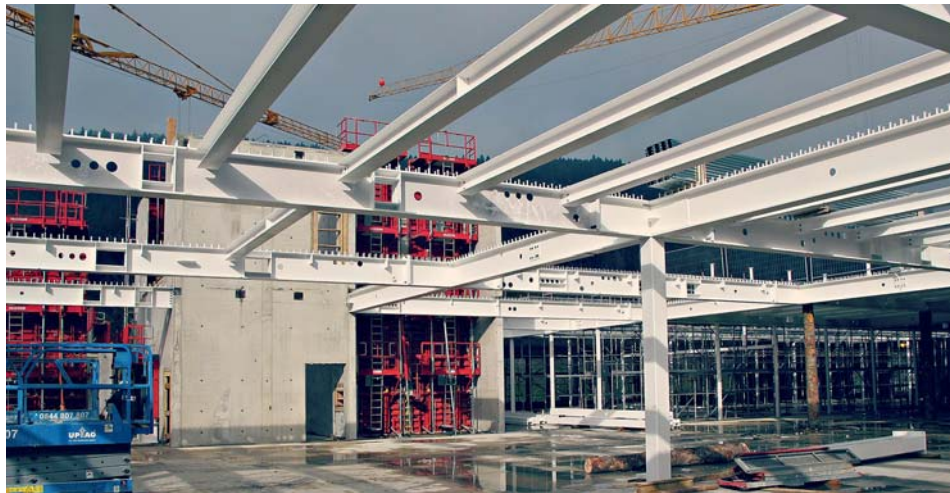
Fig. 3 Montage de la charpente sur atelier. Assembly of the roof structure on the workshop.
