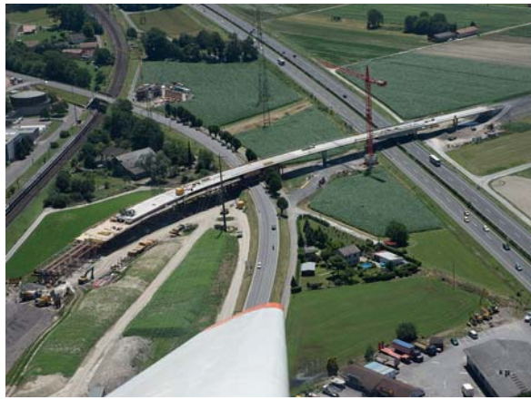
Fig. 8 Vue aérienne du viaduc en construction. Aerial view of the viaduct during construction. (© SR)
